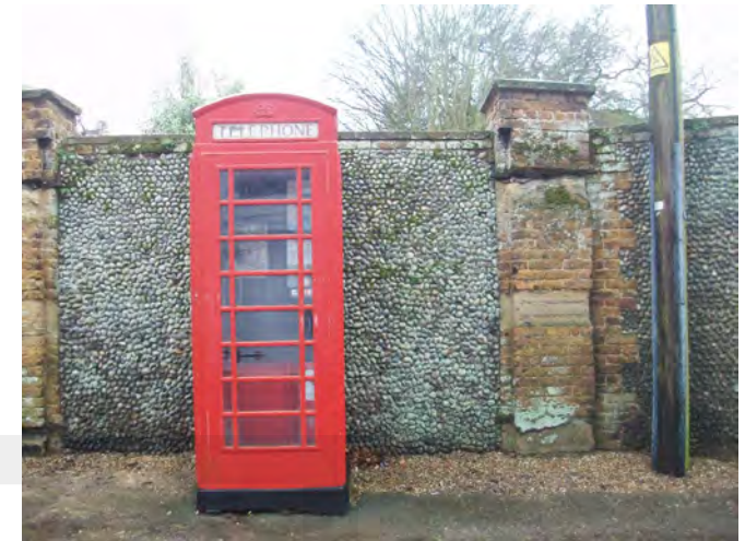
Deteriorating brick work to listed gate piers on the High Street
