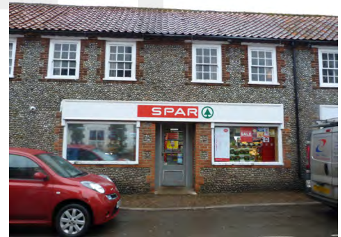
Overly large fascia board to the Spar and garish advertisements
