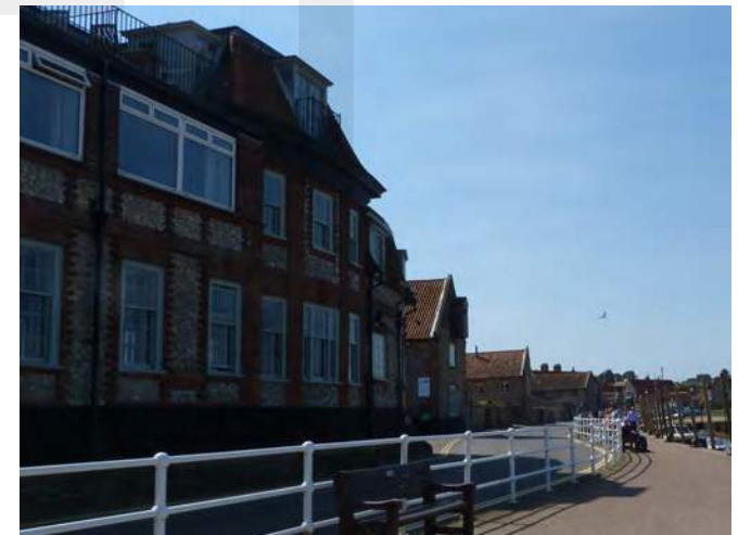
Inappropriate uPVC windows to the first floor viewing gallery at the Blakeney Hotel
