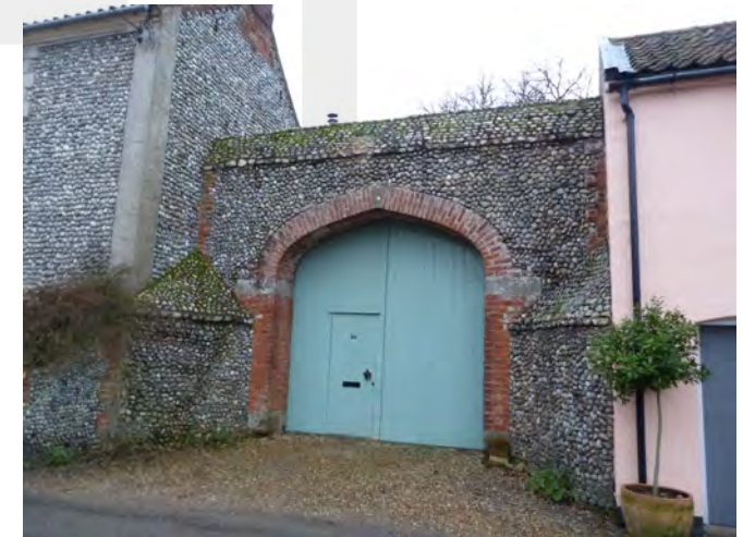
Moss and vegetation starting to build up on flint walls
