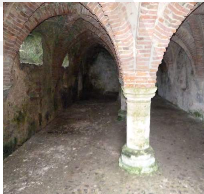
Interior of the Guildhall showing signs of damp
